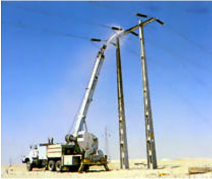
Figure 1: Live line insulator washing of a transmission line.
